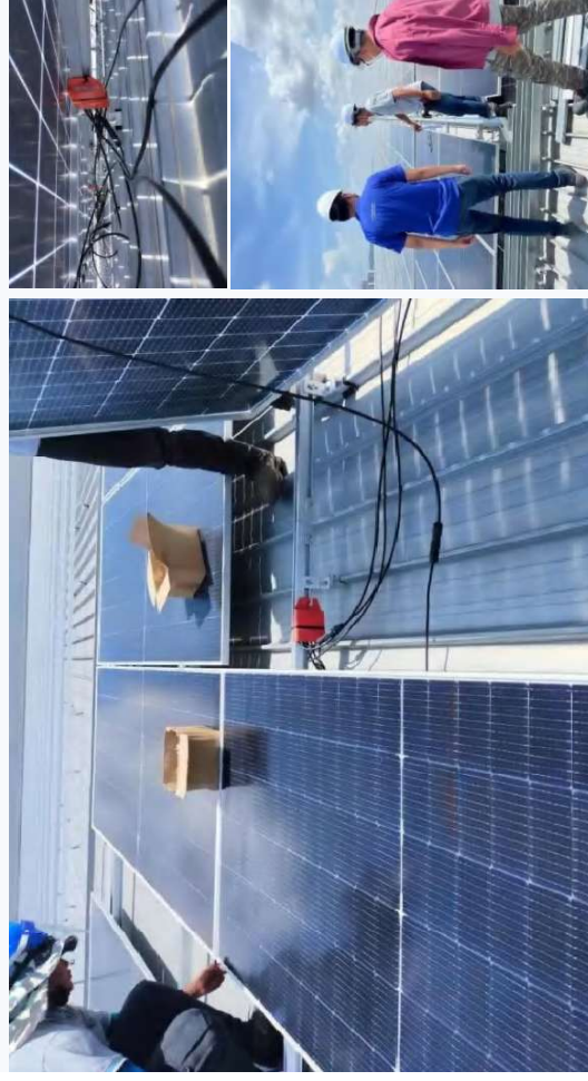
CASE STUDY: 2MW Commercial Rooftop Project in Malaysia
